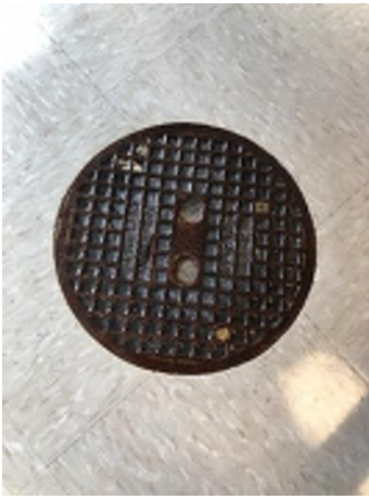
In-Floor Lab Waste Neutralizer
