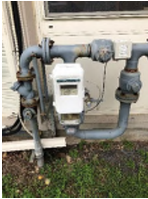
Original Building Gas Service
