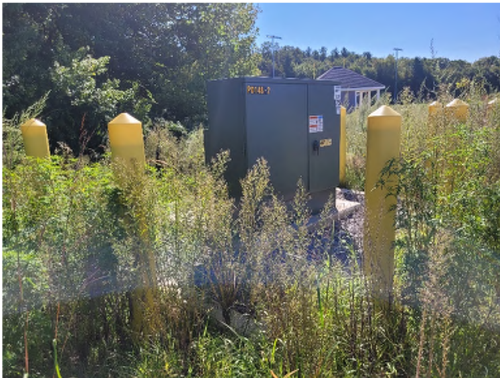
Figure 8: Transformer on the North Side of the Building for Athletic Field Lighting
