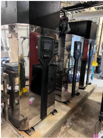
M1 - (3) Camus boilers installed in 2016
