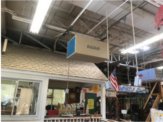
M9 - Air scrubber installed in woodworking room
