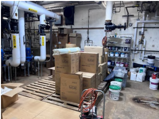
M3 – Location of previously installed oil boiler. The oil boiler and tank have since been removed.
