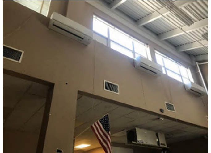
M14 – A/C split units installed in classroom.
