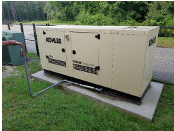
E6 – Kohler 100kw natural gas generator serving 1990s addition
