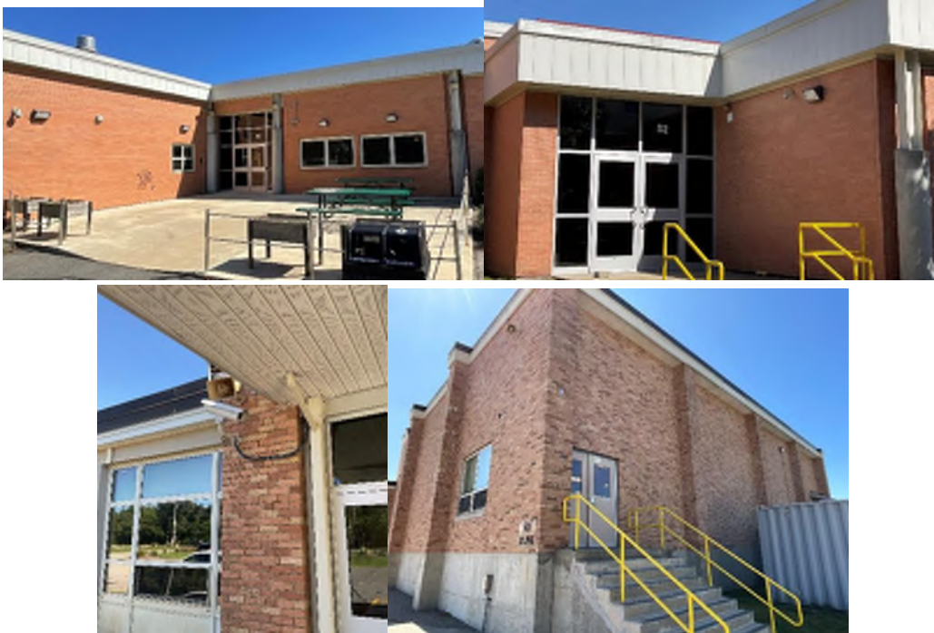
Typical Exterior Cameras
