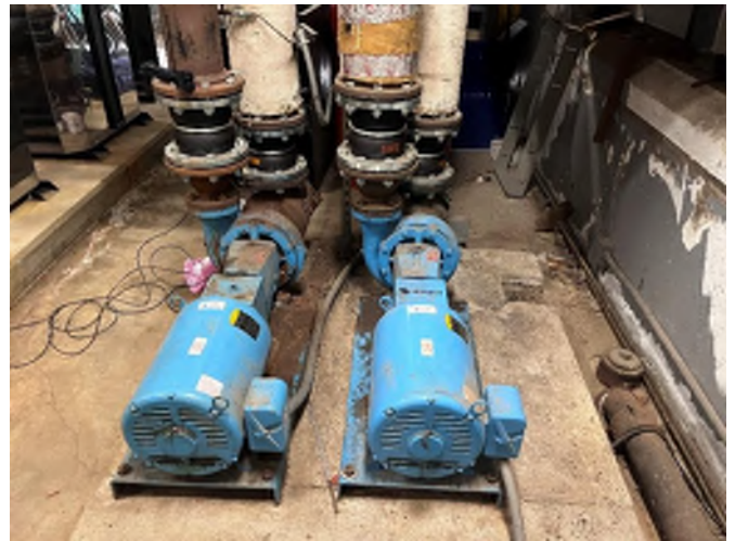
M4 - Hydronic base mounted hot water pumps.
