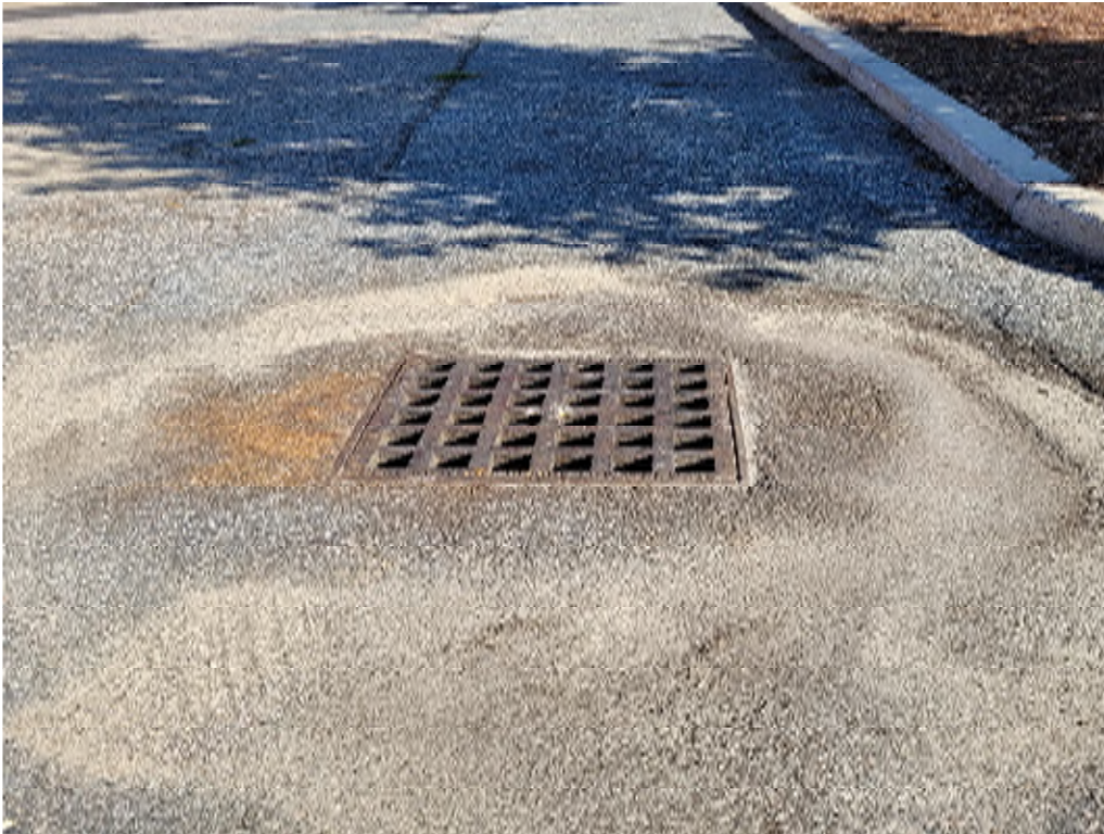
Figure 3: Catch basin at the parking lot at the rear of the school building
