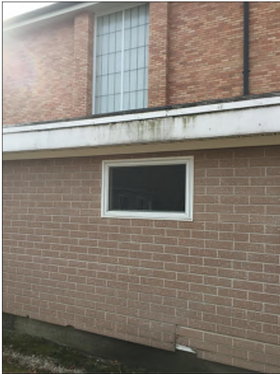
Photo at weight room expansion shows moss growth on existing fascia. Is there an issue with water buildup on the roof?
