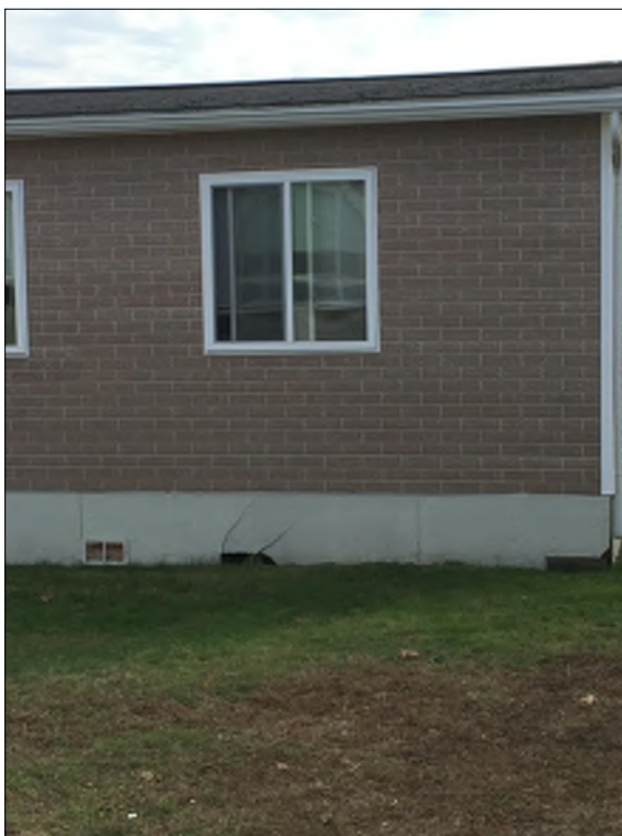
Damage to lower wall sheeting at the modular classroom expansion.
