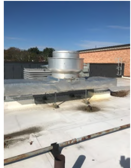
M16 - Kitchen exhaust fan
