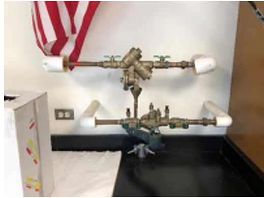
Non-Potable Water Backflow Preventers
