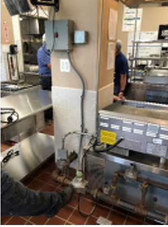
Kitchen Emergency Shut-Off
