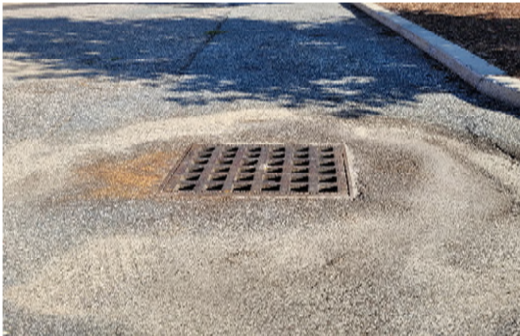
Figure 2: Catch basin at the parking lot at the rear of the school building
