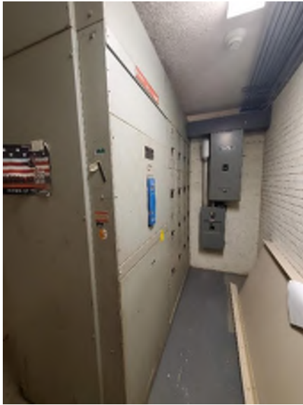
E1 – Original Building electrical service switchboard
