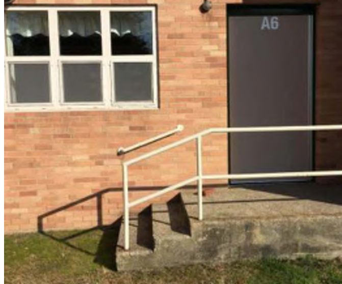
Exterior Stair w/ Noncompliant Handrails
