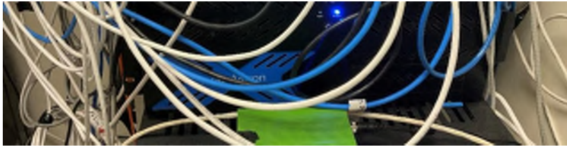
Rack-mounted ExacqVision Server
