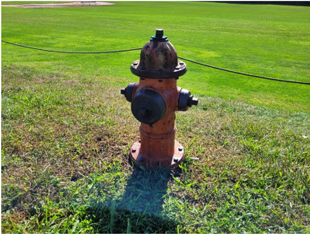
Figure 1: Hydrant Located at the Parking Lot at the Rear of the School Building
