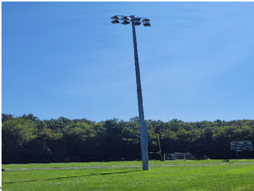
Figure 8: Light Pole at the Athletic Field
