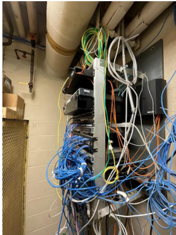
IT Rack – Cafeteria Storage Cage
