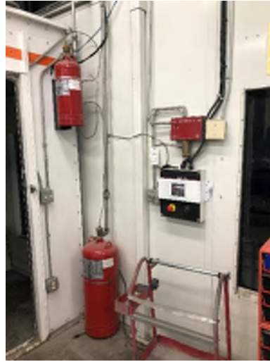
Spray Booth Suppression System
