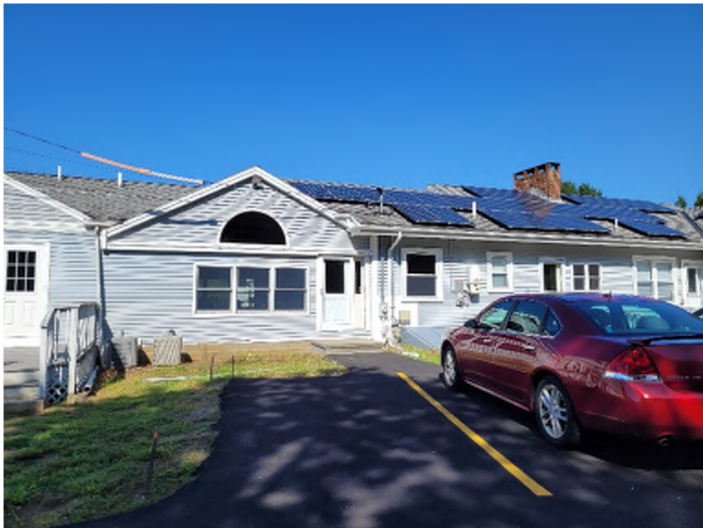
Figure 10: Overhead Electric and Telecom Services for 436 Webster Street
