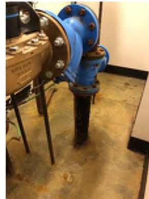
Water Service - 1992 Addition
