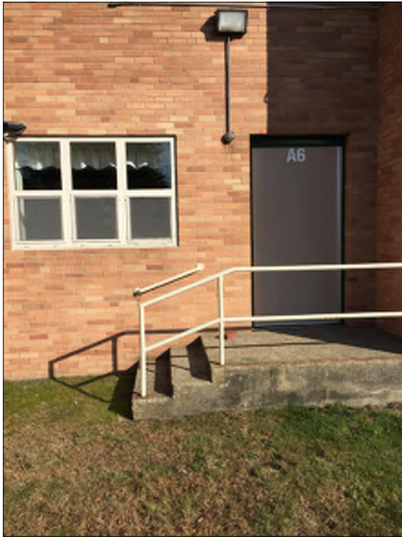
Secondary means of egress from the cafeteria is not considered accessible.
