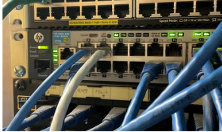
Network Switch Mounted in Main IT Rack
