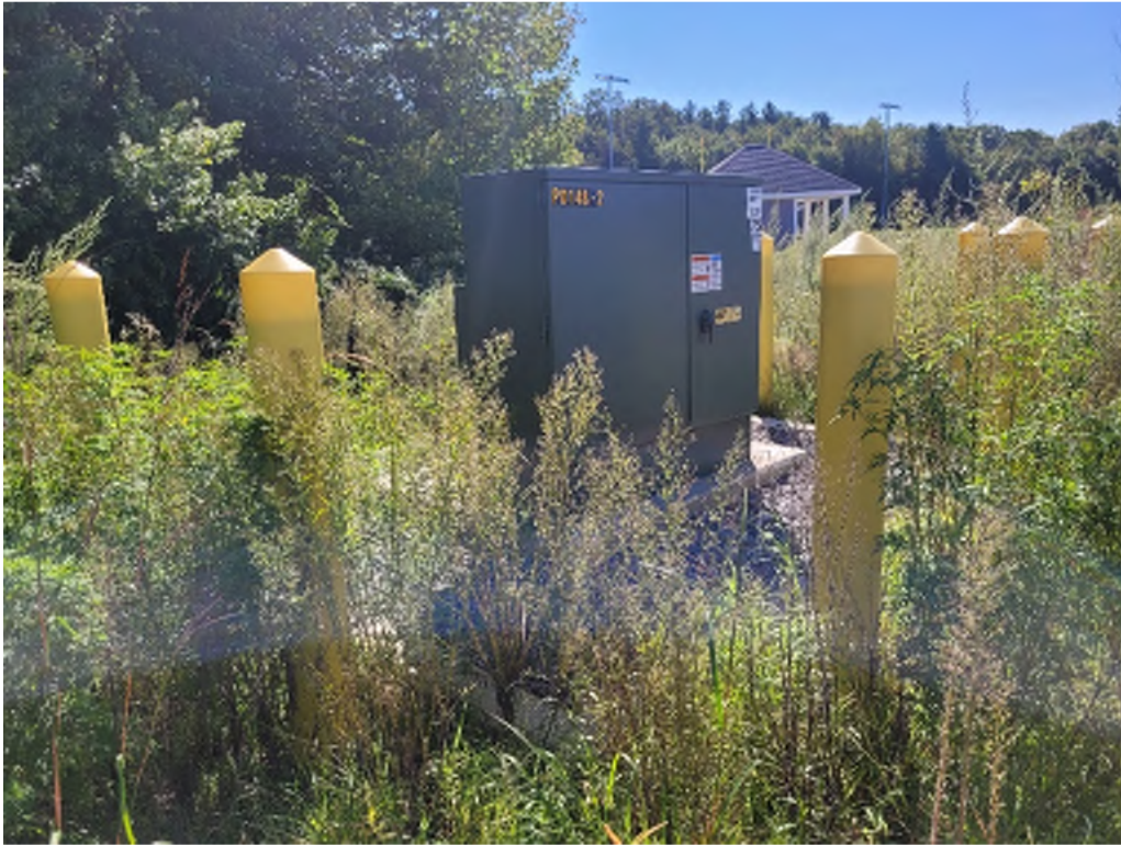
Figure 9: Transformer on the North Side of the Building for Athletic Field Lighting
