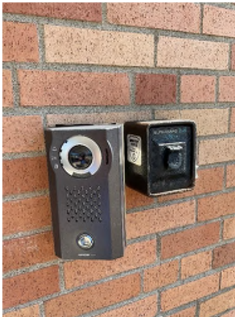
Main Entry Intercom
