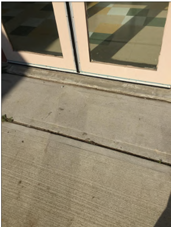
Bump in concrete at back egress doors to the "courtyard" area - may need to be leveled for access.
