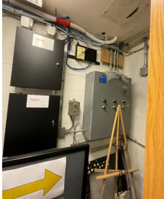
Main Access Control Panel – Main IT Room
