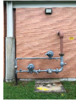
1992 Addition Gas Service
