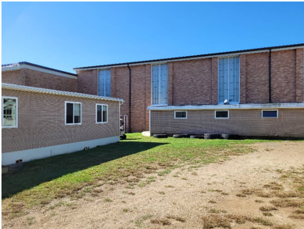
Figure 6: Typical Roof Leaders Connecting to Closed Drainage System
