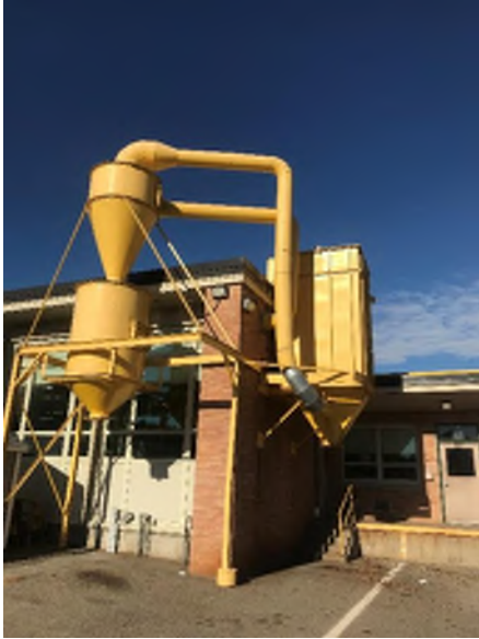
M17 - Dust collector on exterior of building
