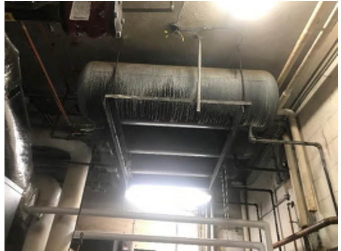
M2 - Ceiling hung expansion tanks
