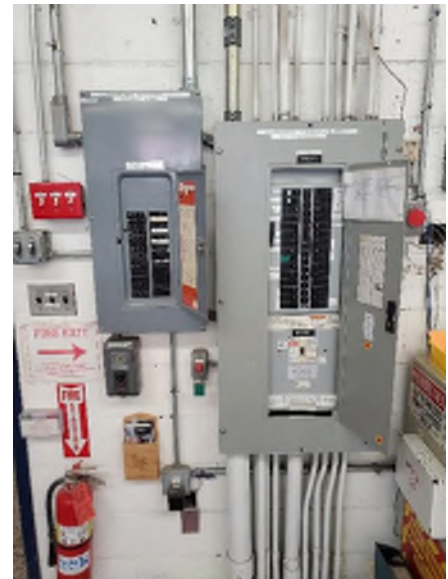
E4 – Branch circuit panelboards in vocational shop area from 1990s renovation
