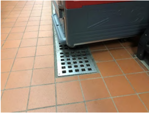
Kitchen Trench Drain
