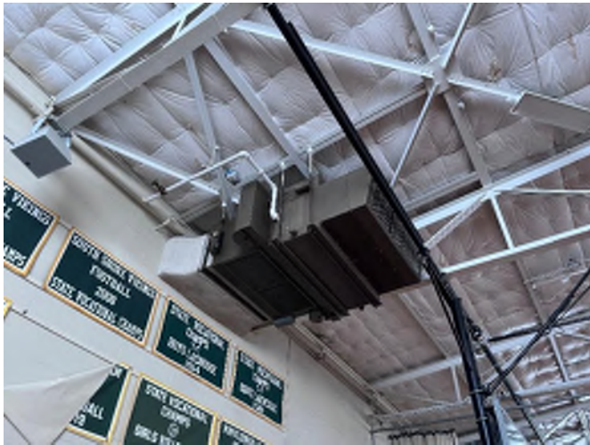
M15 - Typical ceiling suspended fan coil unit. Two units serve gymnasium
