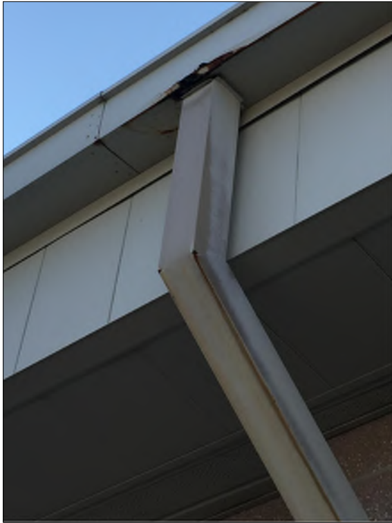
Gutter and downspout at 1992 addition - need to repair damaged fascia. Gutters and downspouts are starting to rust out.
