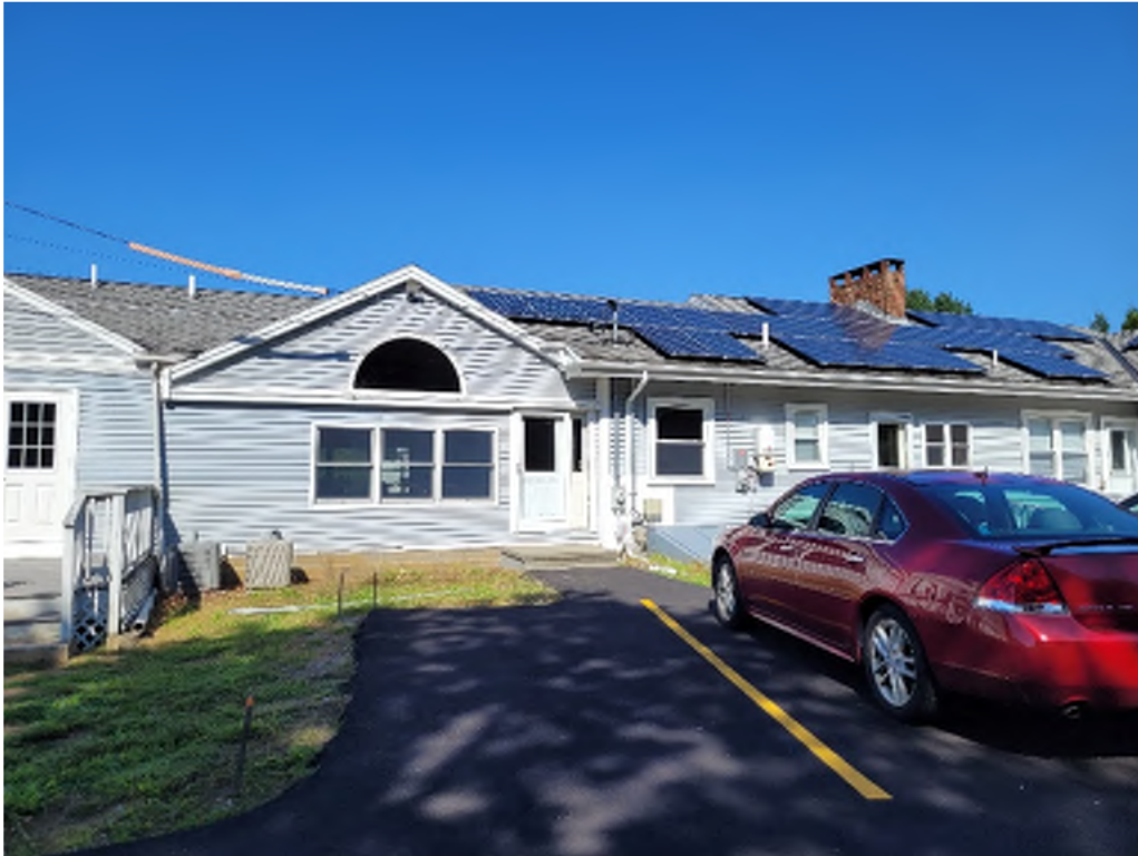
Figure 9: Overhead Electric and Telecom Services for 436 Webster Street
