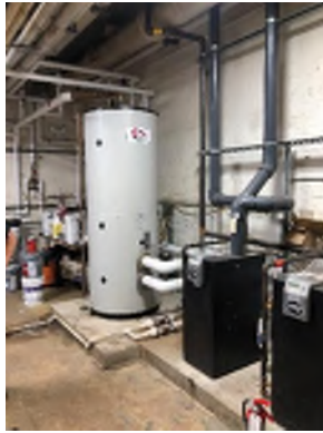
Water Heaters and Storage Tank
