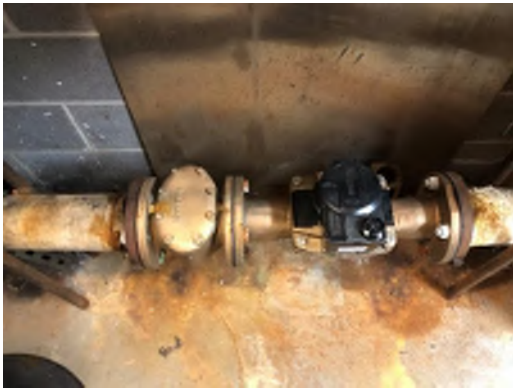
Water Service - Original Building
