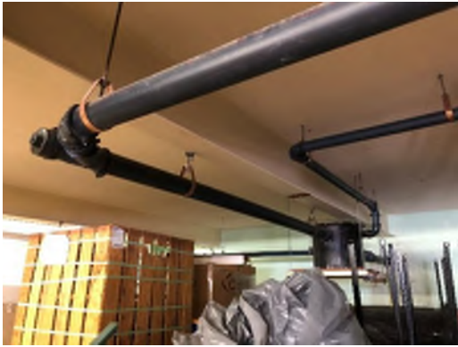
Lab Waste and Neutralizing Tank
