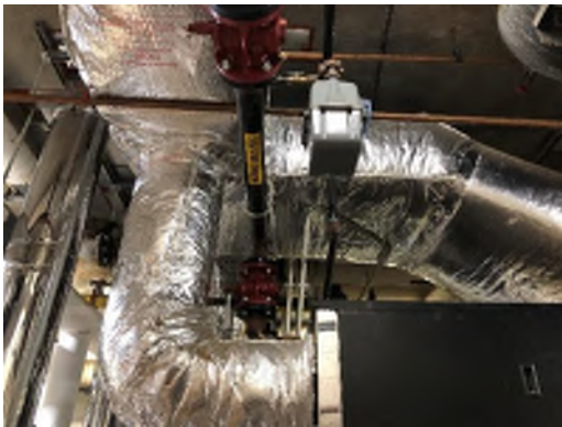
Combustion Air Ducting
