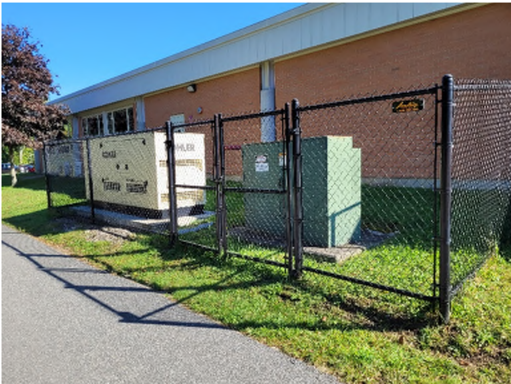
Figure 6: Transformer and Generator on the South Side of the School Building
