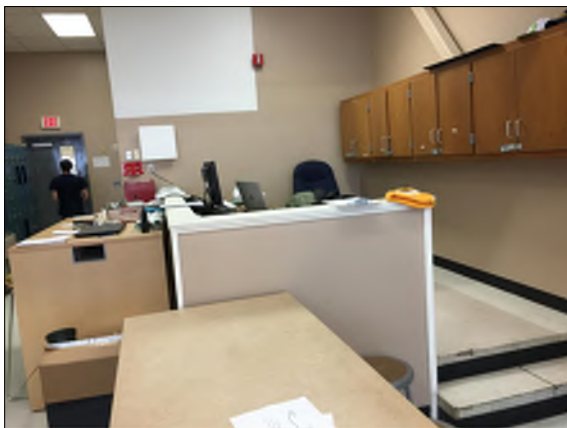
Elevated teachers areas, located in several shop areas (such as automotive and electrical shops), are not considered accessible and should be replaced.
