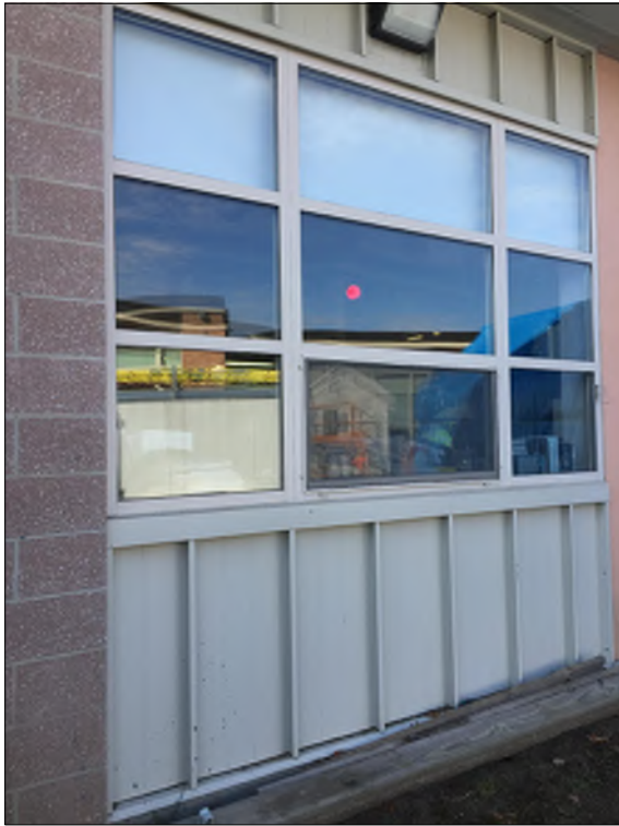
Typical window assembly at the 1992 addition - windows above with operable sections and metal wall panels below.
