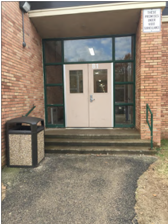
Main Student Entrance doors by student parking lot. Entrance is not considered accessible.
