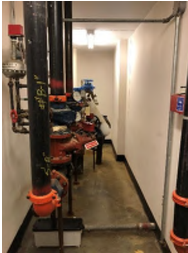
Sprinkler System Riser
