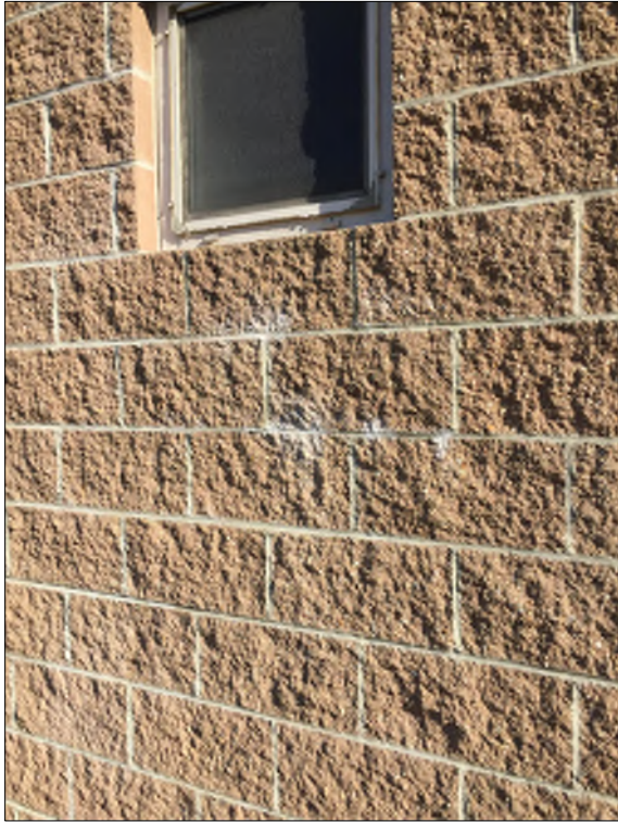
There were some minor spots of efflorescence noted in the 1992 addition.
