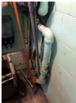
Waste and Vent Piping
