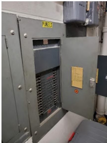
E3 – Branch circuit panelboard from original building construction
