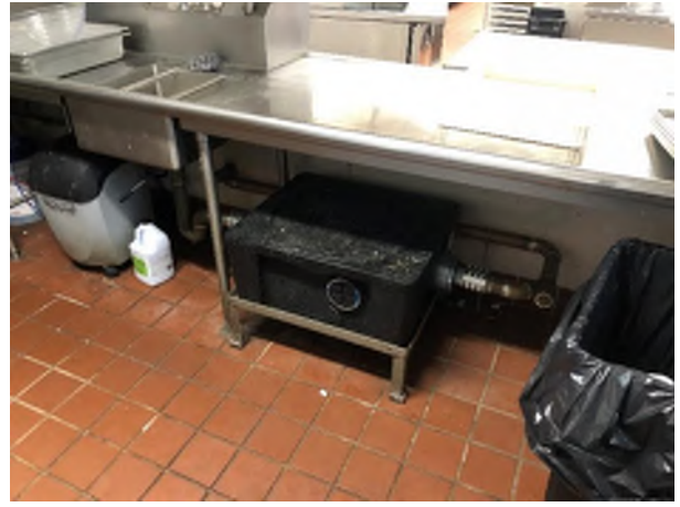
Sink Drain & Grease Interceptor
