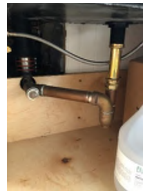
Copper and No-Hub Waste Piping
