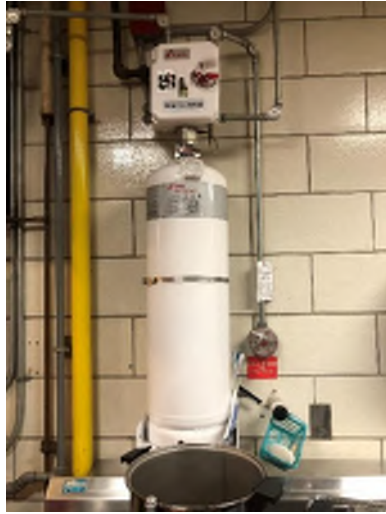
Hood Suppression System
