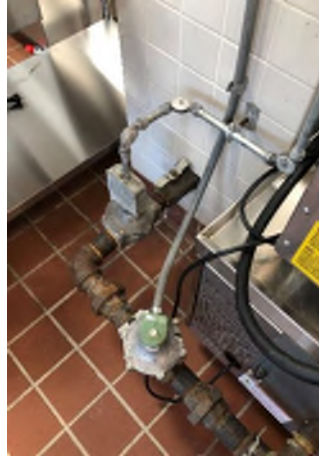
Kitchen Emergency Gas Valve
