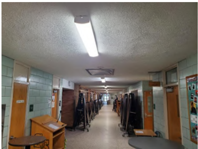
E7 – Typical LED replacement bulbs in fixtures within the original building
