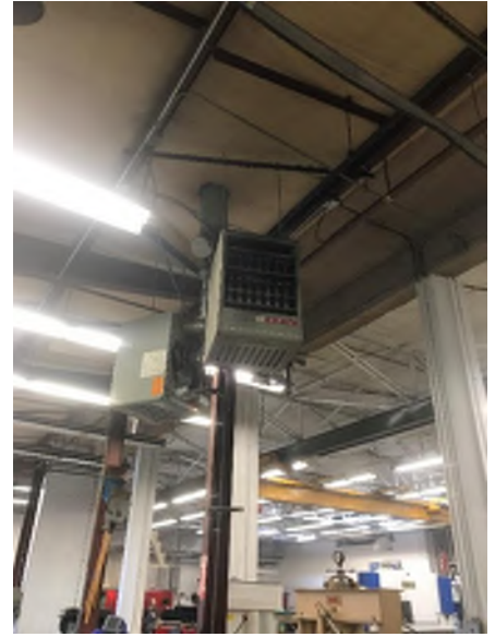
M19 - Ceiling suspended unit heaters
