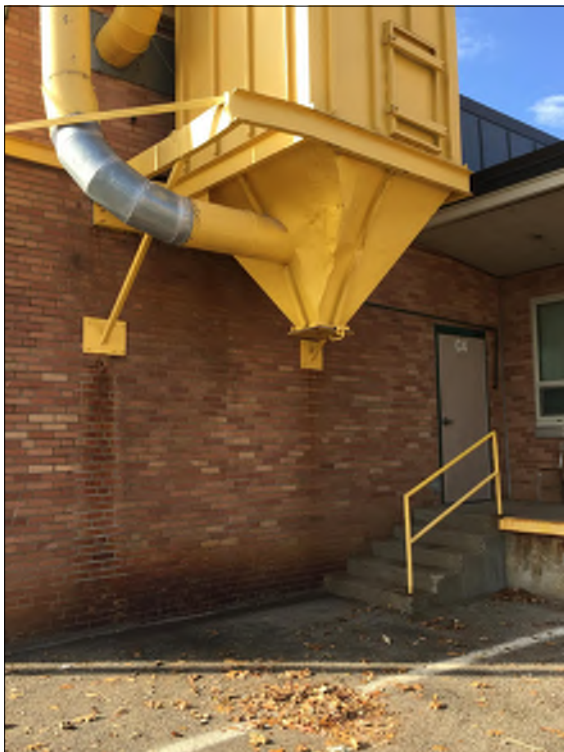
Damage to section of dust collector - hit by trucks in the loading dock area.
