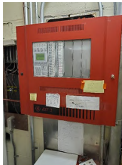
E8 – Edwards fire alarm control panel
