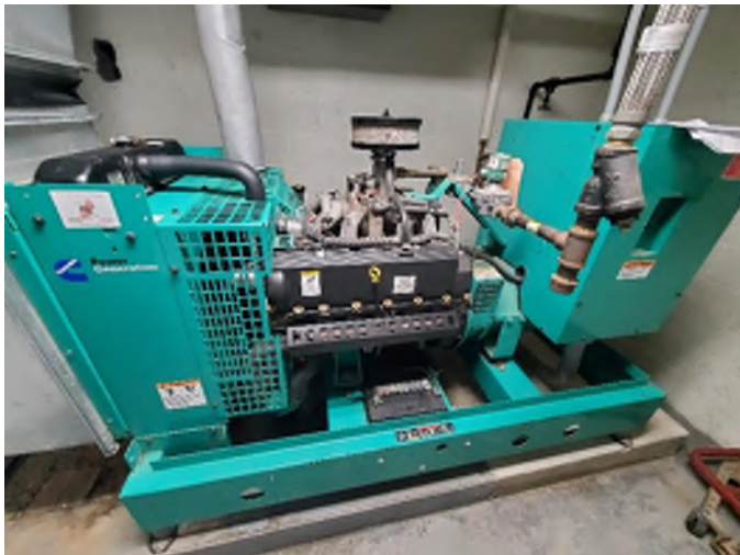
E5 – Cummins 60kw natural gas generator serving original building
