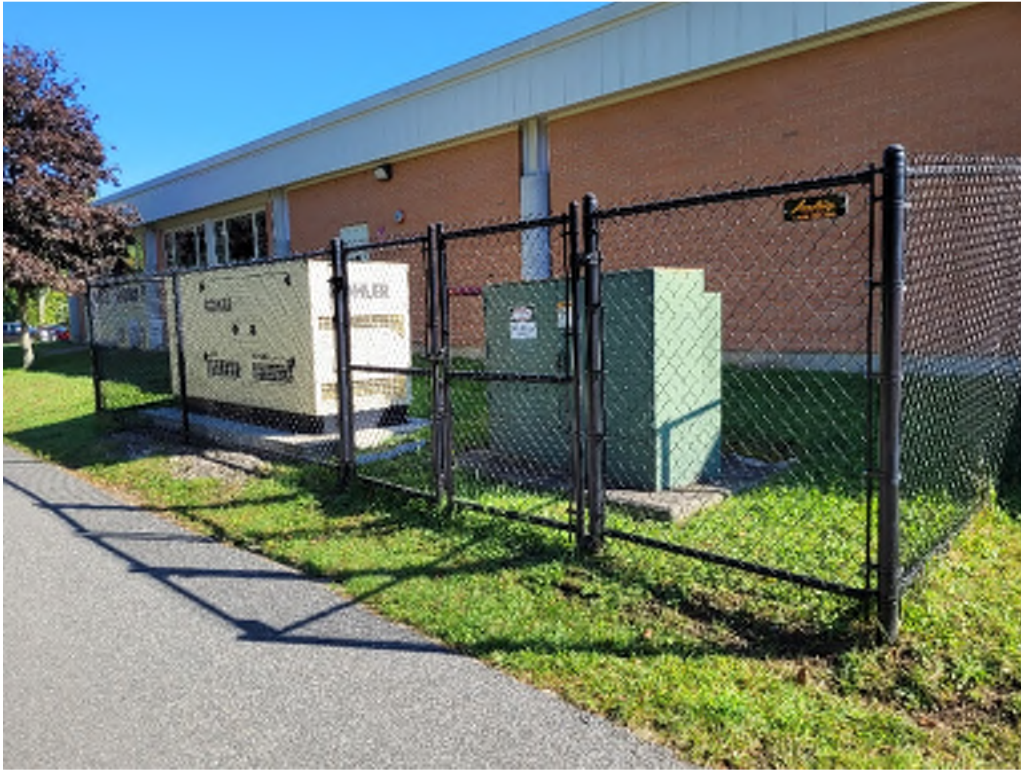
Figure 7: Transformer and Generator on the South Side of the School Building.
