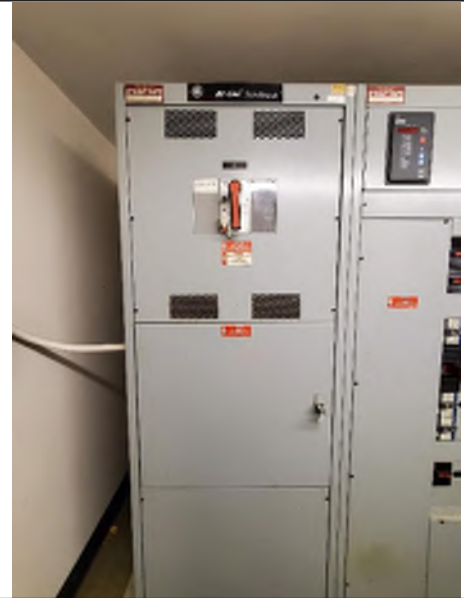
E2 – 1990s addition electrical service switchboard
