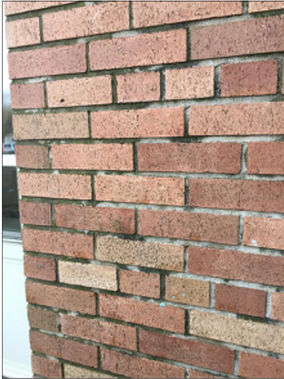
Evidence of moss growth on brick pier near main entrance - water runoff from canopy above
