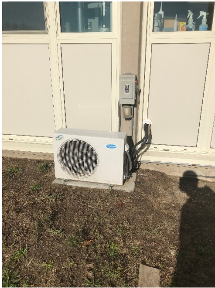
M13 - Outdoor condensing unit for indoor VRF wall mounted split unit
