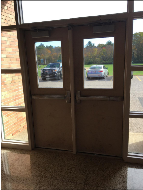
Pair of doors at egress at a pair of 2'-8" doors which are not considered accessible. Doors should be replaced with one leaf at least 3'-0" wide.
