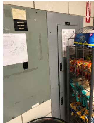
E20 – Kitchen Panels
