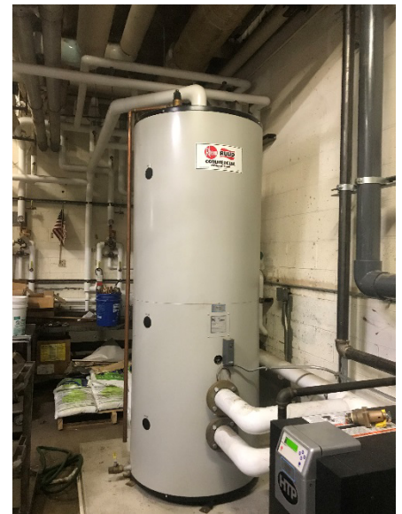
PFP12 – Domestic hot water storage tank
