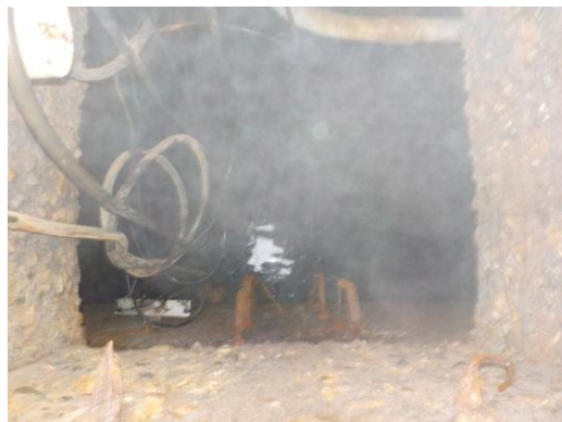
Figure 7 – View of Pump Chamber Manway with Power & Control Wiring
