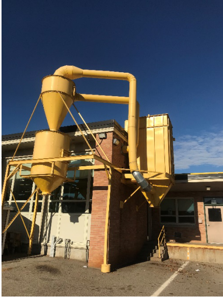
M17 - Dust collector on exterior of building
