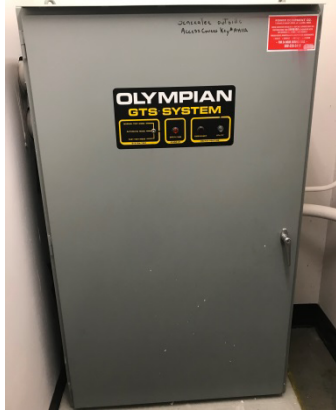
E9 – Building Addition Transfer Switch
