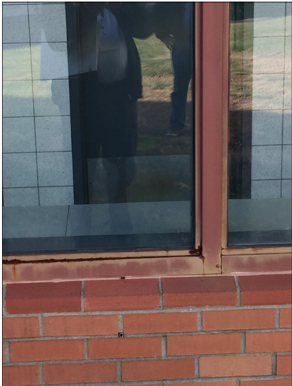
Evidence of rusting at the windows frame in the 1992 addition.
