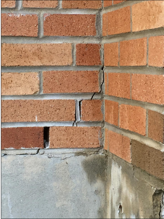
These appear to be some settlement cracks which should get patched.
