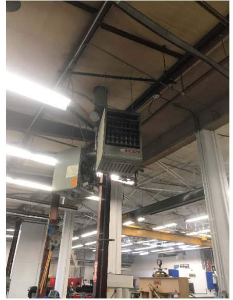
M19 - Ceiling suspended unit heaters
