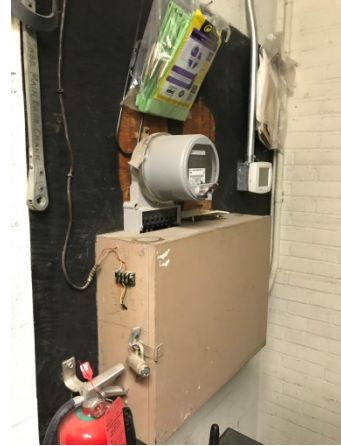
E2 – CT Cabinet and Meter
