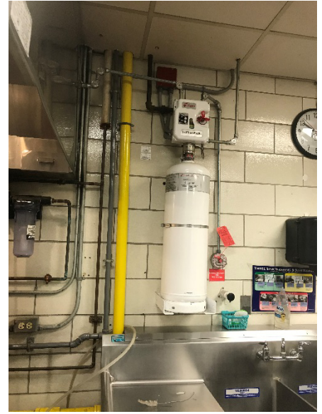
PF14 – Kitchen hood fire suppression system
