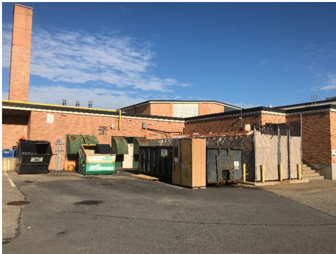
M3 - Exterior above grade oil tank
