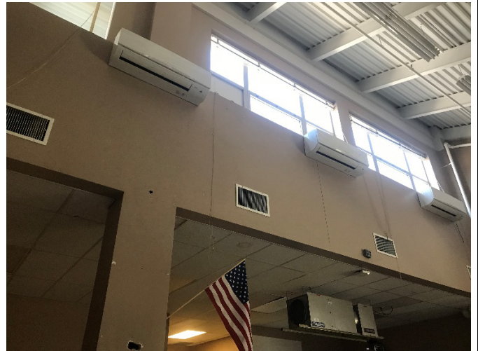
M14 - A/C split units installed in classroom.
