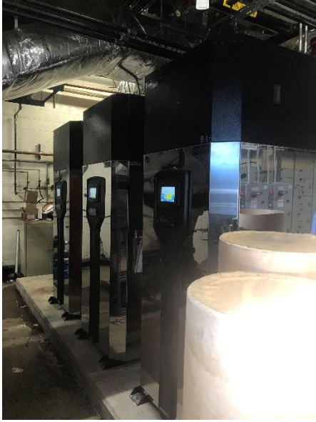
M1 - (3) Camus boilers installed in 2016
