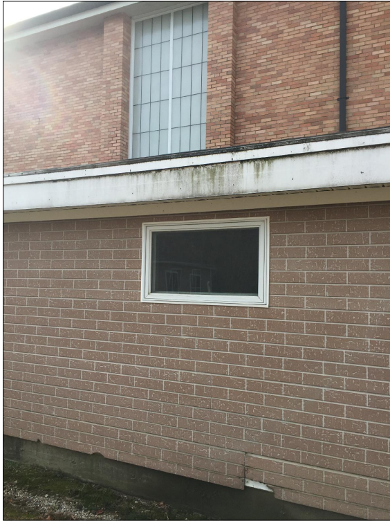
Photo at weight room expansion shows moss growth on existing fascia. Is there an issue with water buildup on the roof?
