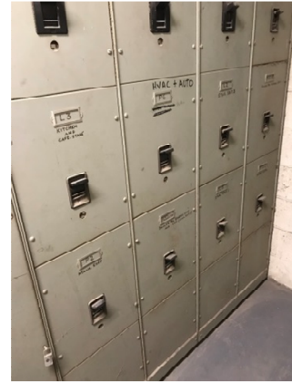
E4 – Electrical Distribution
