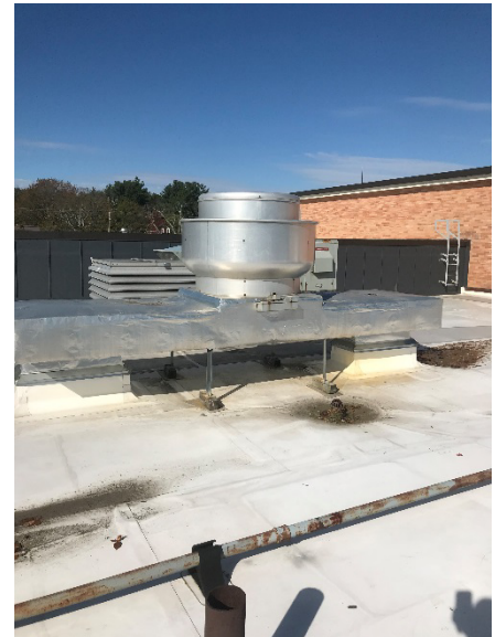
M16 - Kitchen exhaust fan
