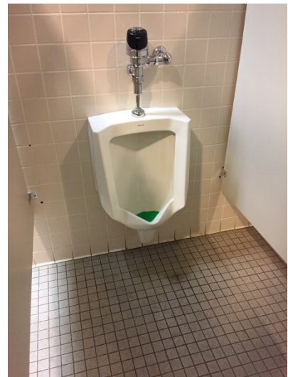
PFP4 – Wall mounted urinal
