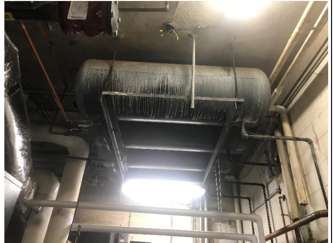
M2 - Ceiling hung expansion tanks
