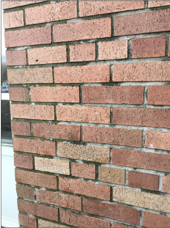
Evidence of moss growth on brick pier near main entrance - water runoff from canopy above
