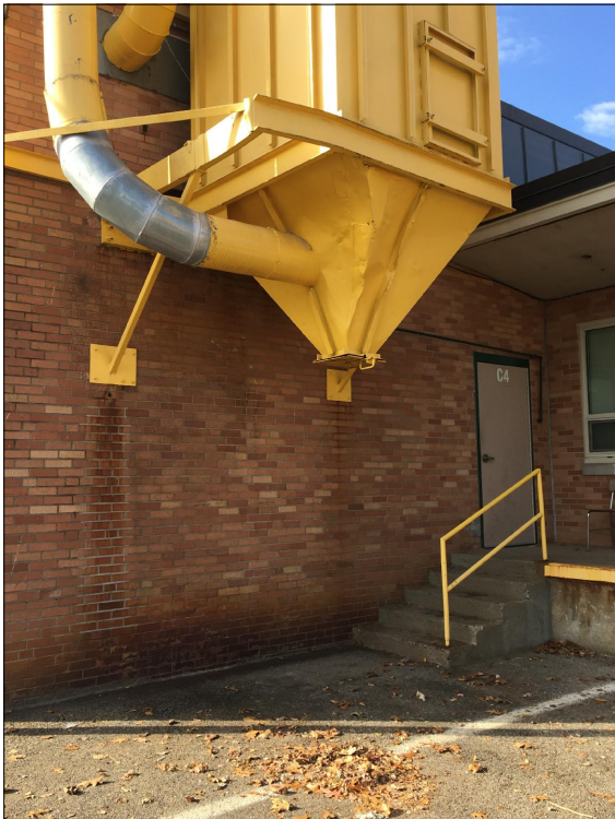
Damage to section of dust collector - hit by trucks in the loading dock area.
