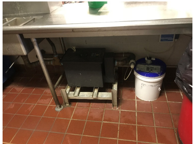
PFP8 – Grease trap mounted below kitchen sink
