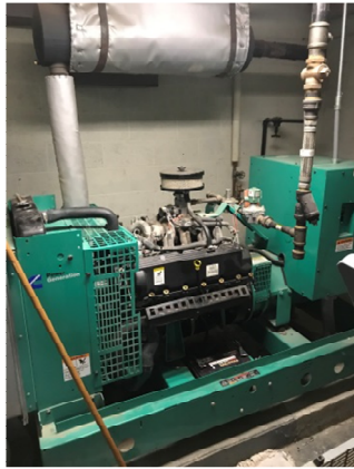
E7 – Original Building Generator
