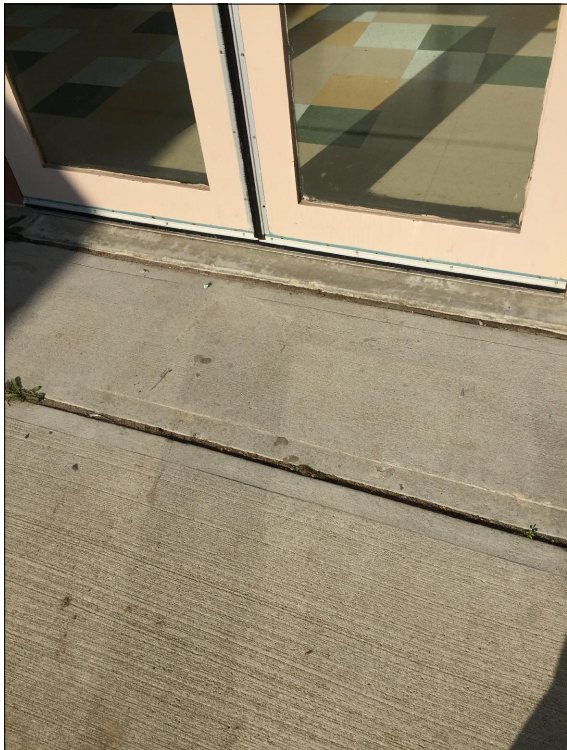
Bump in concrete at back egress doors to the "courtyard" area - may need to be leveled for access.
