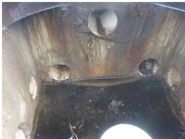
Figure 8 – View of D-box Serving the West Side Soil Absorption System
