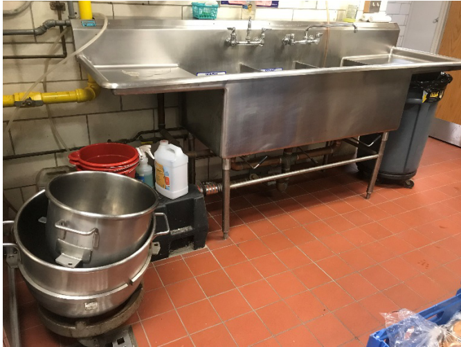
PFP9 – Kitchen 3-bay sink with inline grease trap
