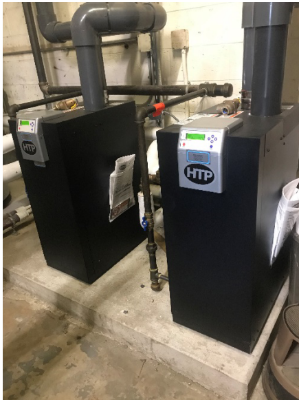
PFP11 – Gas fired domestic water heaters
