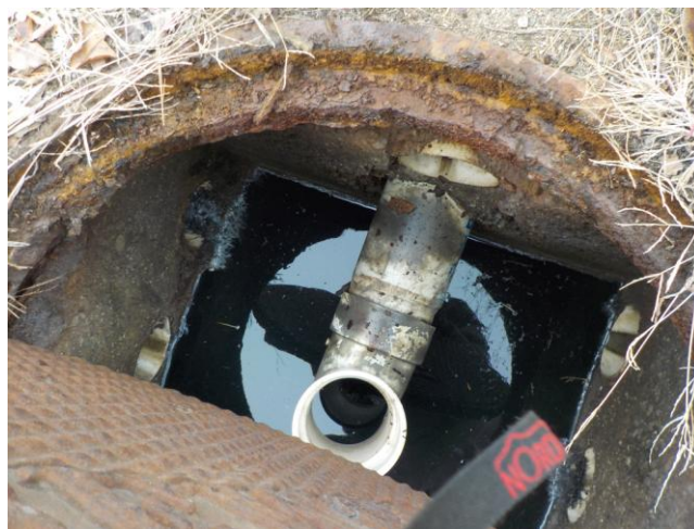
Figure 9 – View of D-box Serving the East Side Soil Absorption System
