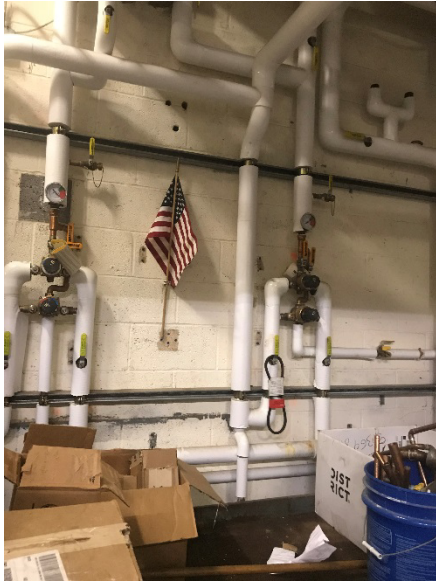
PF13 – Domestic hot water tempering valves
