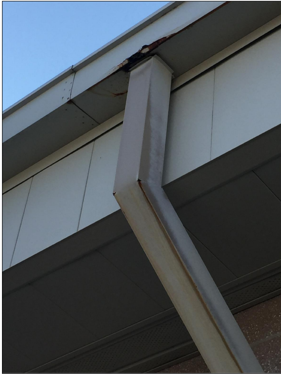
Gutter and downspout at 1992 addition - need to repair damaged fascia. Gutters and downspouts are starting to rust out.
