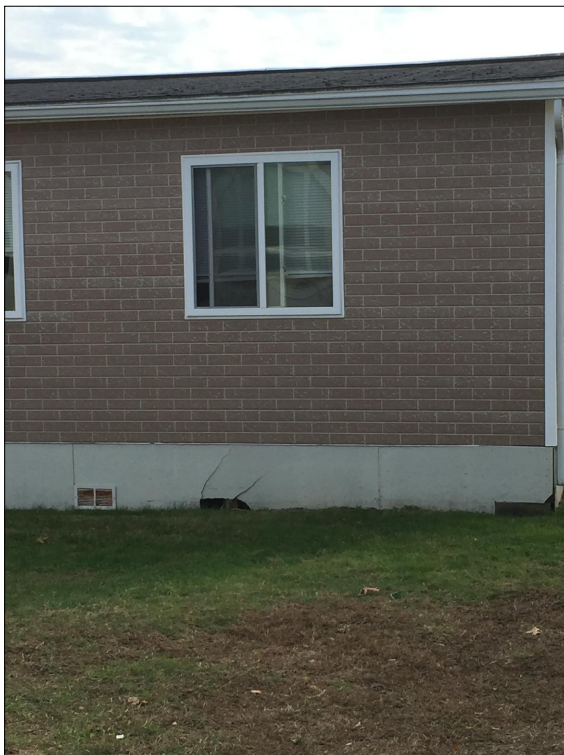
Damage to lower wall sheathing at the modular classroom expansion.
