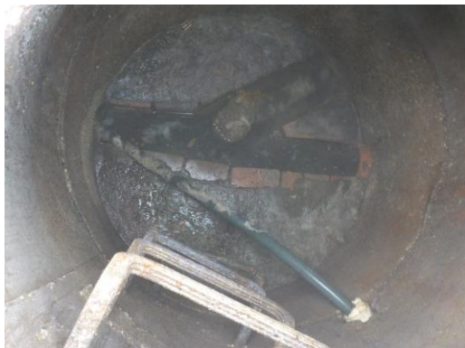
Figure 5 – Sewer Manhole with what is Believed to be the Force Main from the Concession Stand
