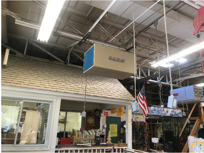
M9 - Air scrubber installed in woodworking room
