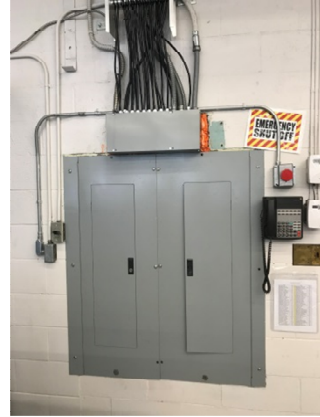
E22 – Typical Shop Panel
