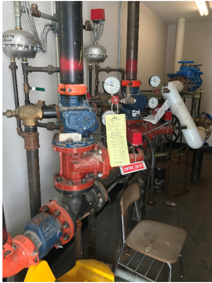
PFP1 – Fire Protection and domestic water service serving 1992 addition
