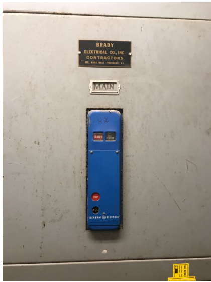
E1 – Original Building Main Disconnect Switch
