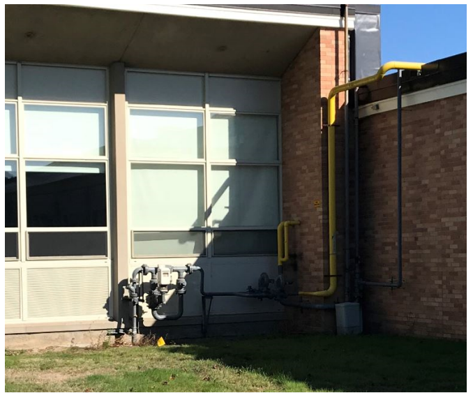
PFP2 – Natural gas service 1962 building
