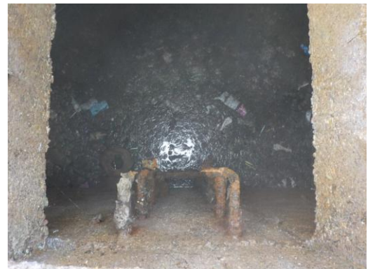
Figure 6 – View of Septic Tank Manway with Corroded Steps
