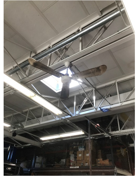
M10 - Typical paddle fan throughout some shops
