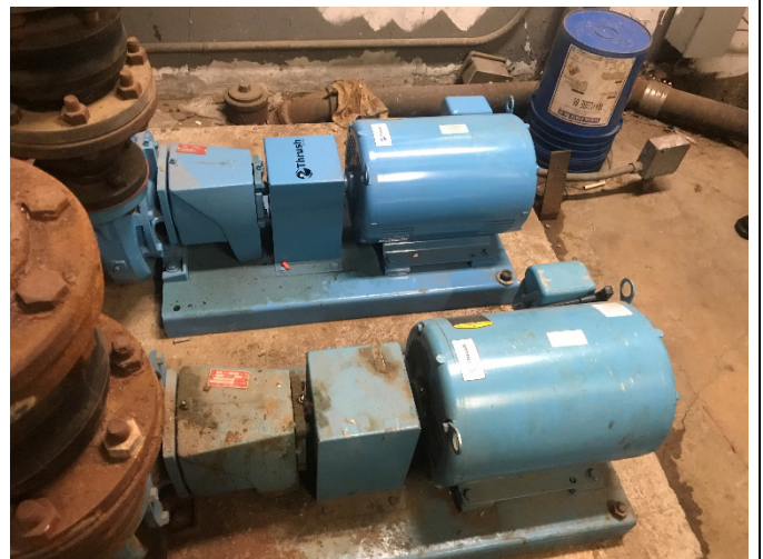
M4 - Hydronic base mounted hot water pumps.
