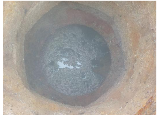
Figure 4 – Grease Trap Showing only Light Accumulation of FOG
