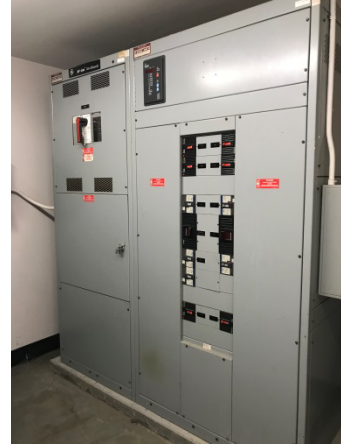
E6 – Addition Electrical Service
