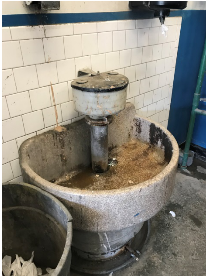
PFP7 – Floor mounted sink in shop
