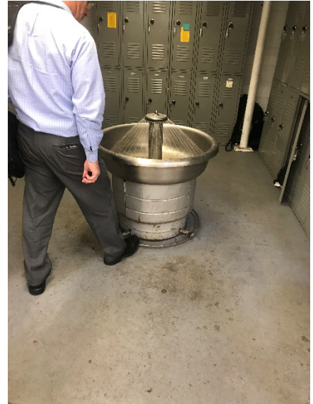
PFP6 – Floor mounted sink in shop
